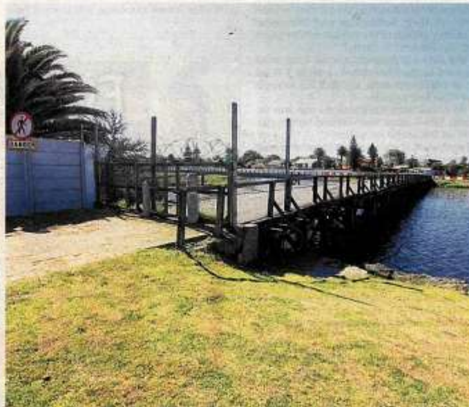
The City of Cape Town will soon commence with a detailed design for the restoration of the historic wooden bridge in Milnerton.
