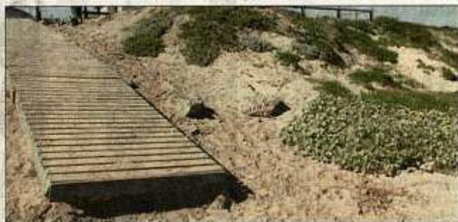
■ Illegal structures on the coastal property in Sunset Beach have led to the City declaring the area part of the Table Bay Nature Reserve.
