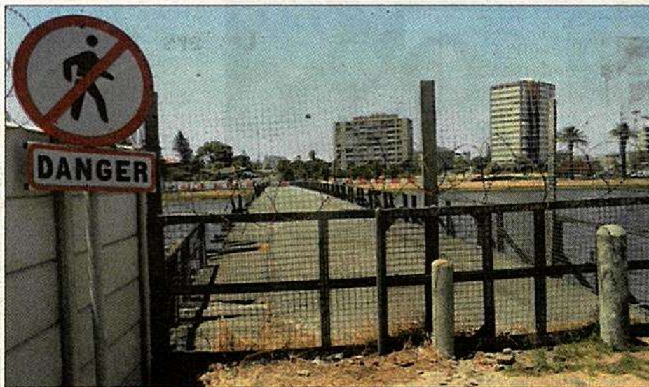
■ The wooden bridge was shut down in 2007 when it was deemed too dangerous to walk on.
